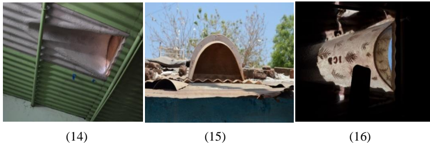
Set D: Ujasiyu – The finalised product installed on the roof (Source: Trivedi, 2014) (Image 14, 15 and 16 – Pre-fabricated FRP product installed on the roofs of the houses; image 16 - embedded leaf patterns visible on the FRP sheets)
