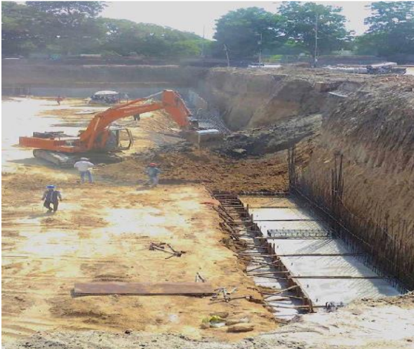
Picture 4.19 Students interacting in a group as team members and monitoring excavation field practicum under the supervision of site supervisors.
