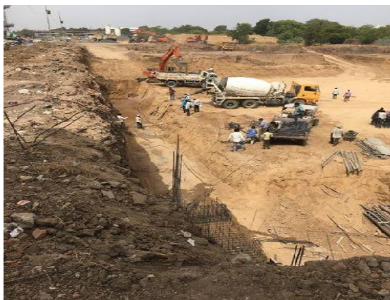
Picture 4.35 Students observing and monitoring the excavated area for reinforcement design of foundation construction
