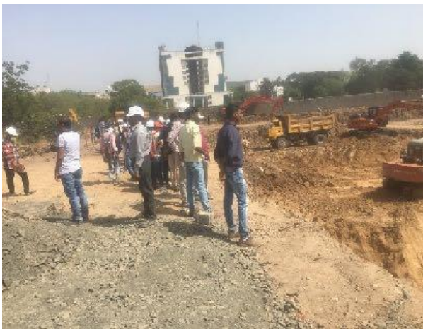
Picture 4.15 Students interacting with team members and site supervisors for excavation field practicum
