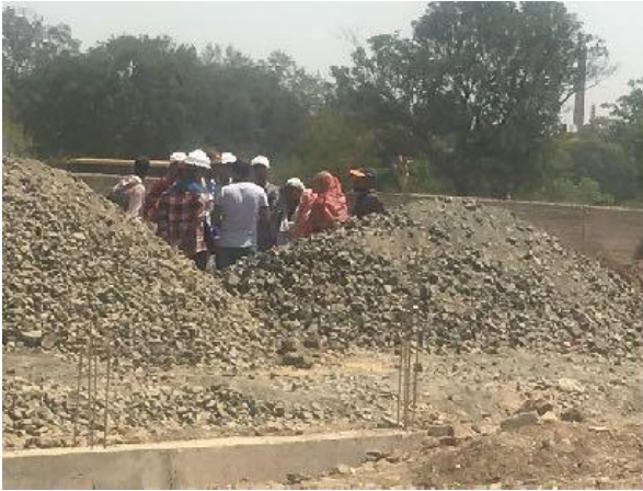
Picture 4.16 Students interacting in a group as team members and ensuring and monitoring excavation field practicum under the supervision of site supervisors.
